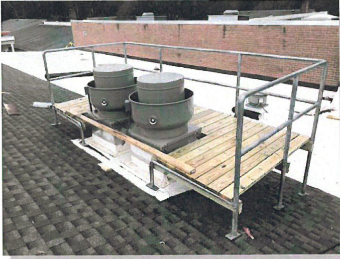
Exhaust Fan Maintenance Platform
