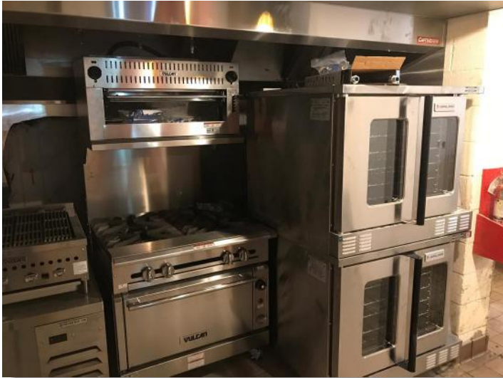
Permanent Kitchen Food Service Hood
