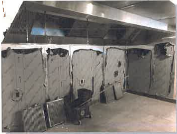
Permanent Kitchen Food Service Hood
