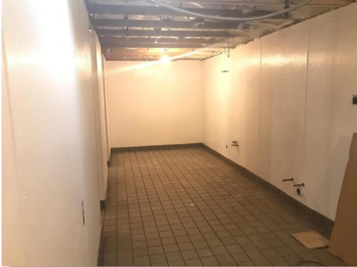
FRP in Permanent Kitchen
